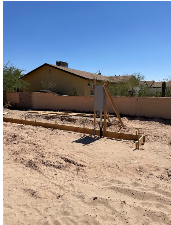
Location of electrical panel (East side of property)
