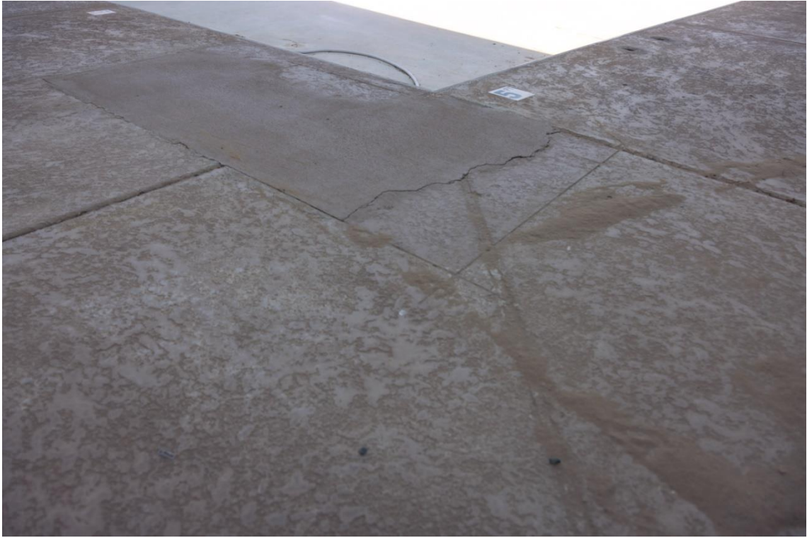
Damage Concrete Surface
