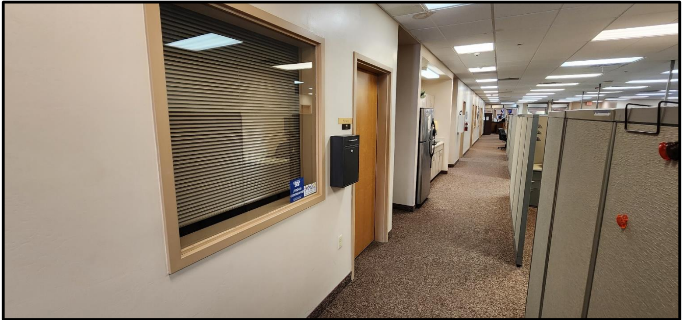
Section 3: Installation of new restroom. On the left: Office will turn into restroom and storage.
