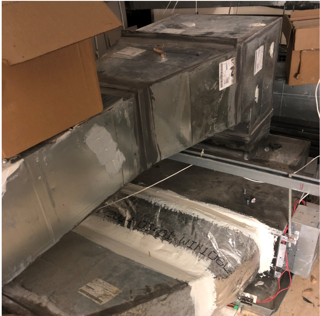
Figure 1: High Loss Elbow into Fan Inlet
