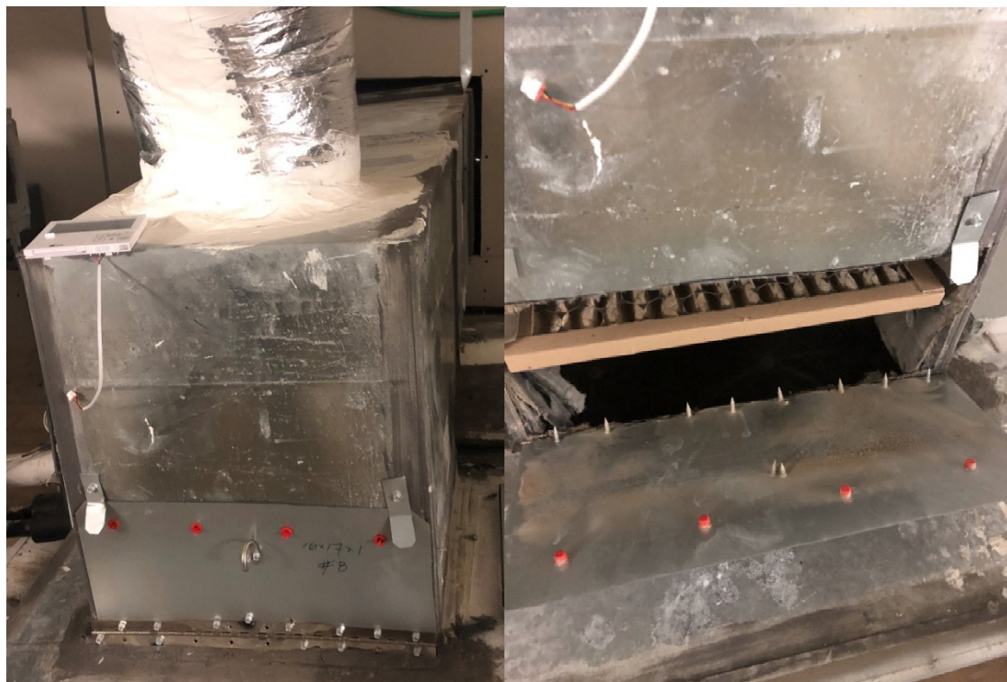
Figure 2: Field-Built Filter Access
