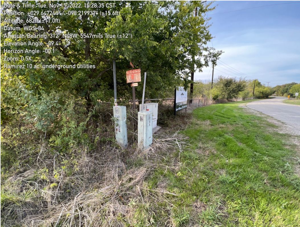
Photo 5. Underground utilities at southeast corner of subject property (Bunker Street on right).
