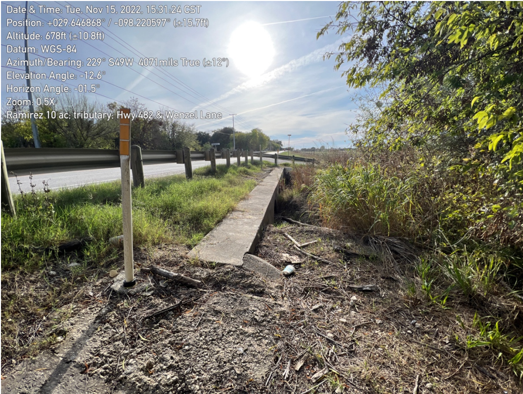
Photo 7. Highway 482 crossing of tributary of Dry Comal Creek (subject property on right).
