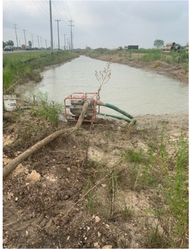
dewatering of trench for installation of gravity main on west side of FM 1518
