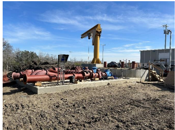
View of lift station site piping pad, wet well, and jib crane
