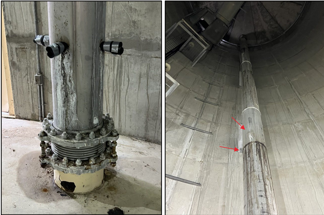
Figure 1. Site Photographs of Leaking Pipes
