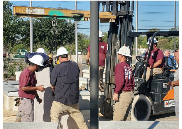
The Parks Maintenance team working to install the new granite fixtures at Veteran's Memorial Plaza.
