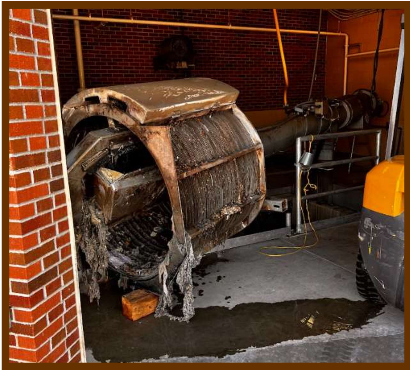
WWTP ROTAMAT PHOTO ATTACHMENTS
