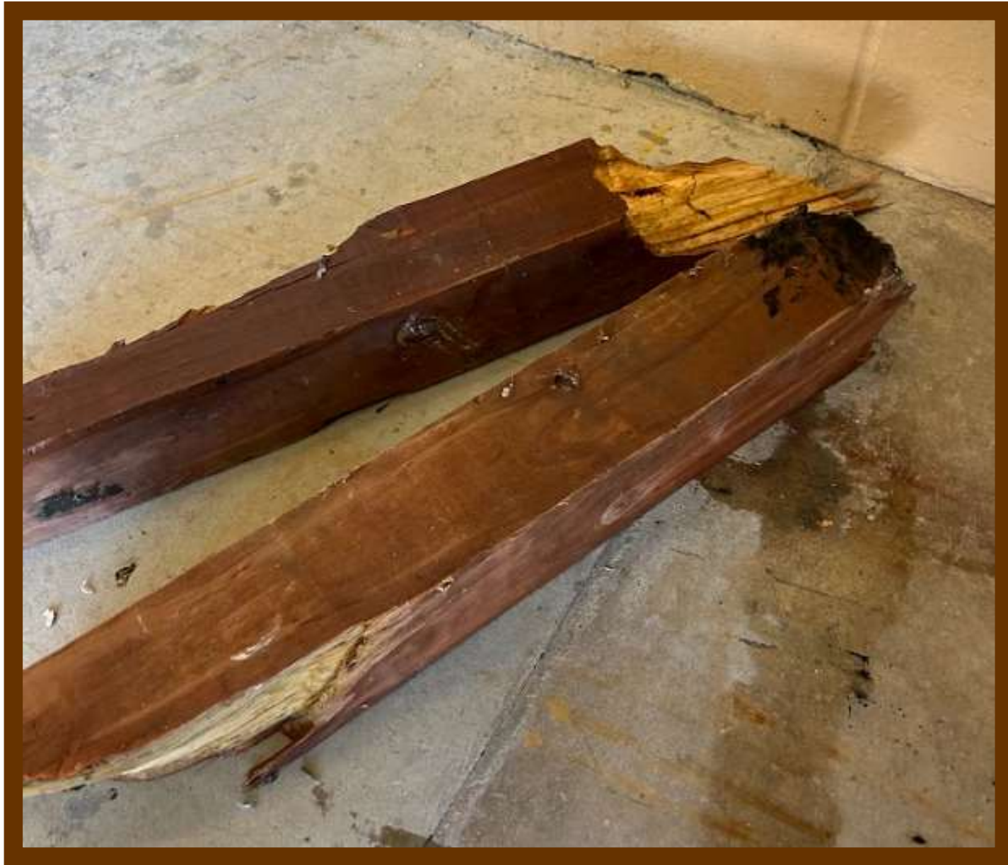
WWTP ROTAMAT PHOTO ATTACHMENTS
