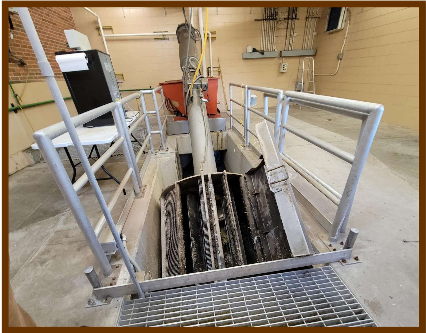
WWTP ROTAMAT PHOTO ATTACHMENTS
