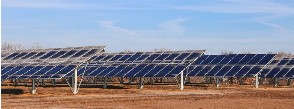
Typical Solar Arrays
