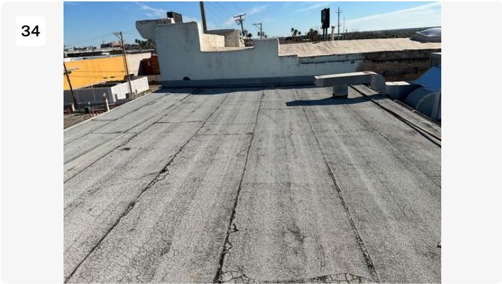
Overview of section of roof with severe wear & tear
