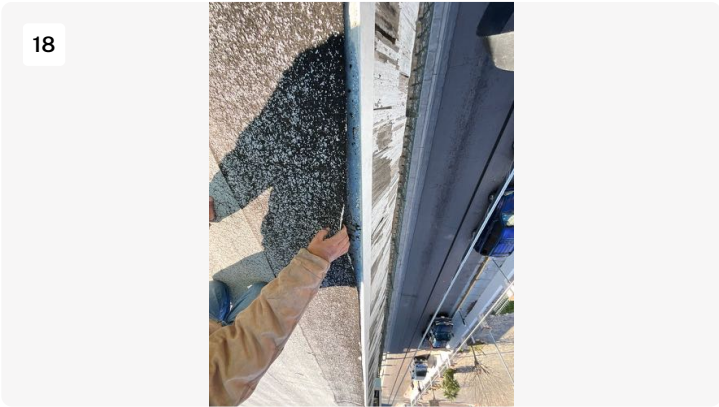
BUR membrane is detaching and coming undone
