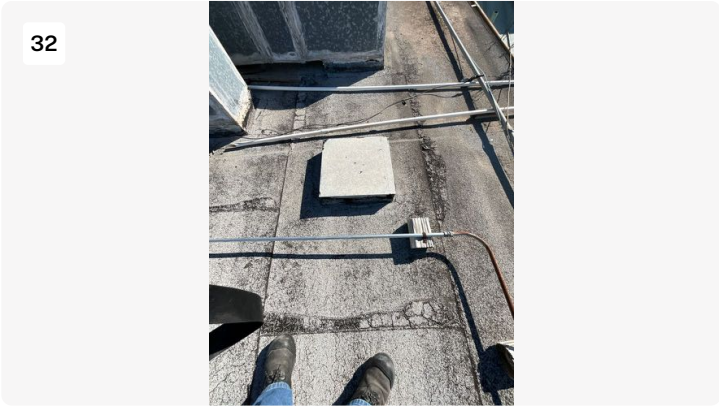
Broken and disconnected PVC pipes
