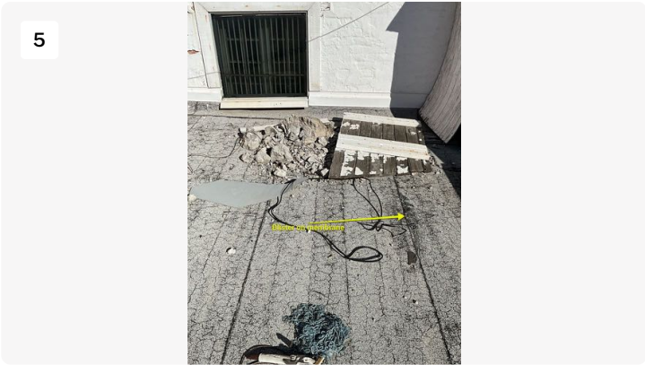
Blister on roof membrane
