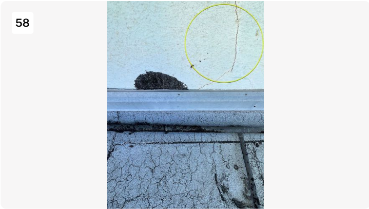
Cracks on parapet wall
