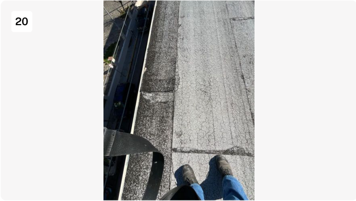
BUR membrane severely worn is observed
