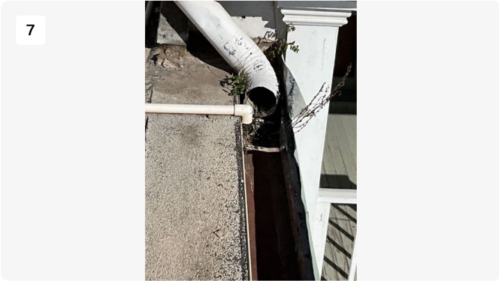
Rust observed on gutter
