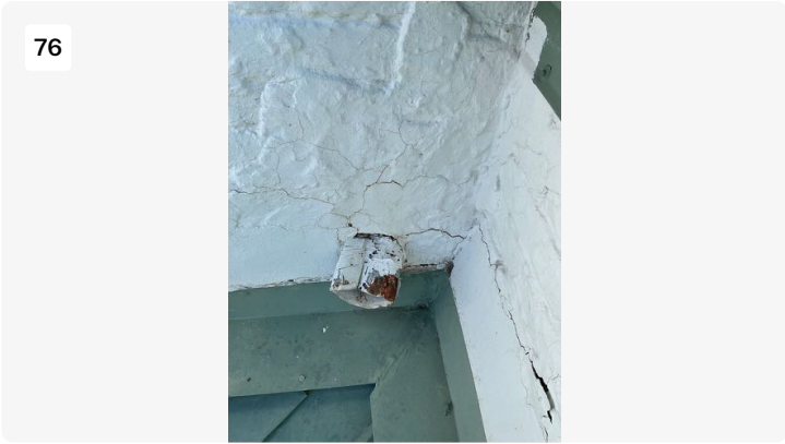
Cracking & peeling at parapet wall observed
