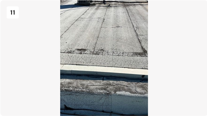
Severe wear & tear on roofing membrane
