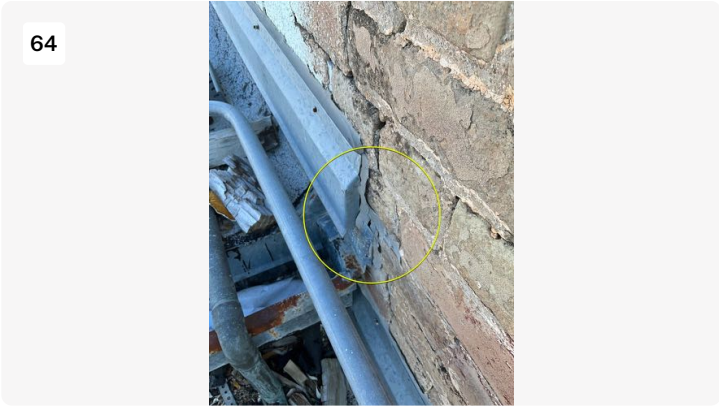
Counter flashing is detaching from the brick wall
