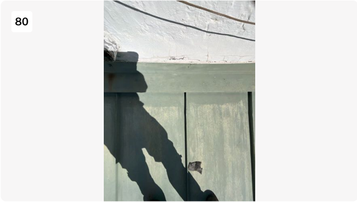
Voids on counter flashing sealant
