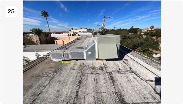
Poorly installed AV vent penetration, correct flashing re- quired
