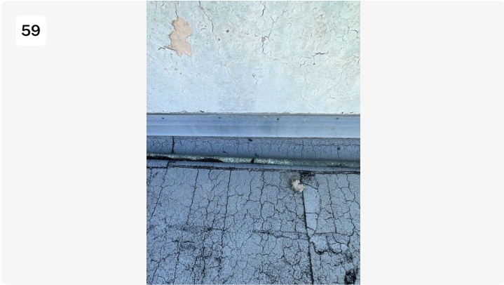
BUR membrane is detaching and coming undone at the base
