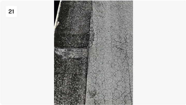
Base flashing coming undone
