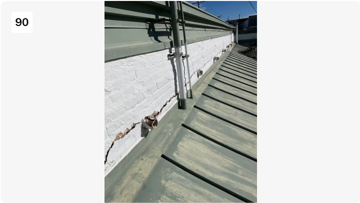
Cracks on parapet wall at SS metal section
