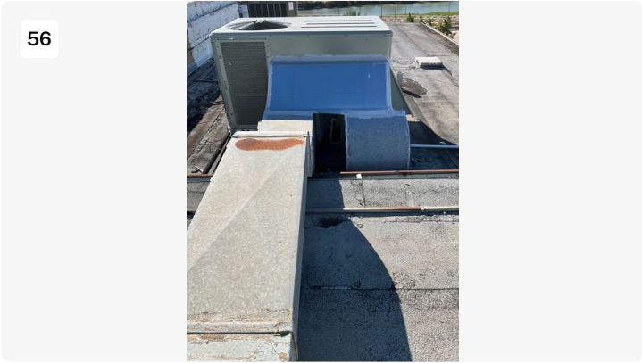
AC unit overview
