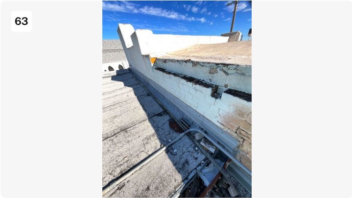
Exposed brick wall along with a excessive amount of trash and debris
