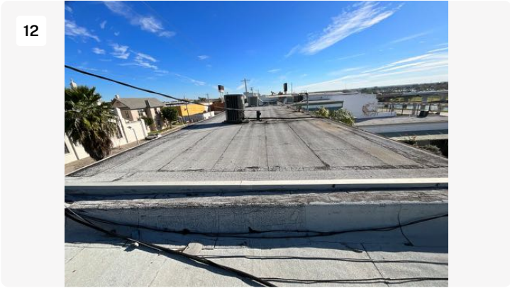
Severe wear & tear on roofing membrane
