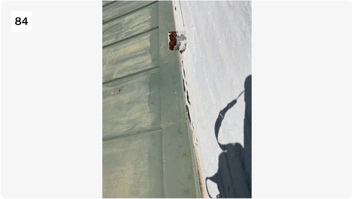
Voids on counter flashing sealant
