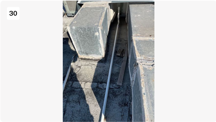
AC duct penetration observed with previous repair material
