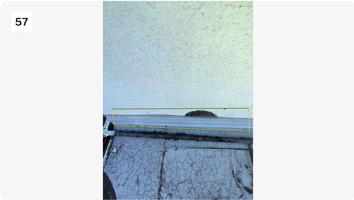
Counter flashing is detaching from parapet wall due to missing fasteners
