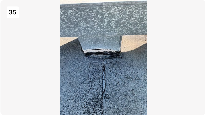
BUR membrane coming apart at roof penetration
