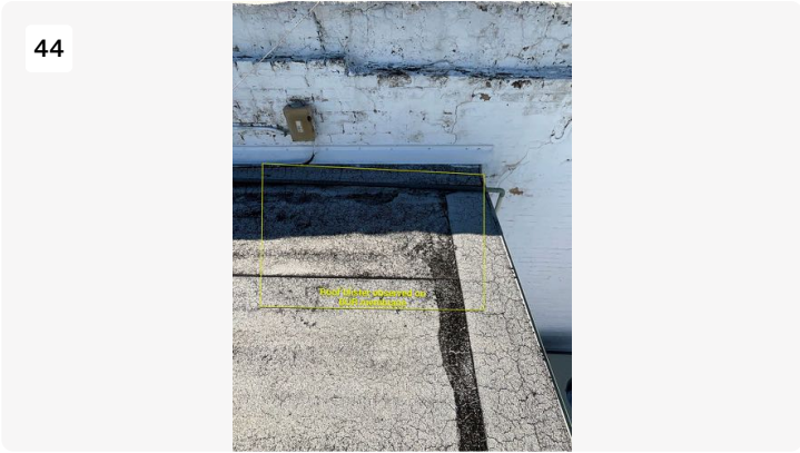
Roof blister observed on BUR membrane
