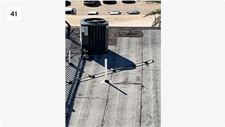
Previous repairs observed on BUR membrane
