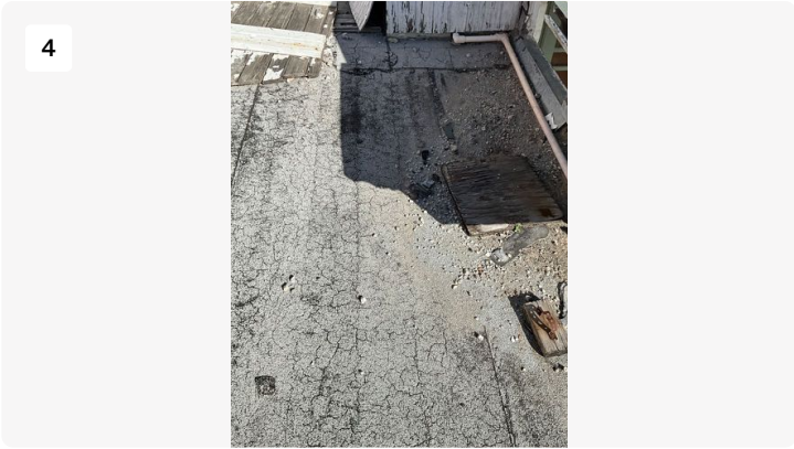
Debris on roof
