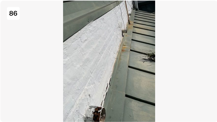
Voids on counter flashing sealant
