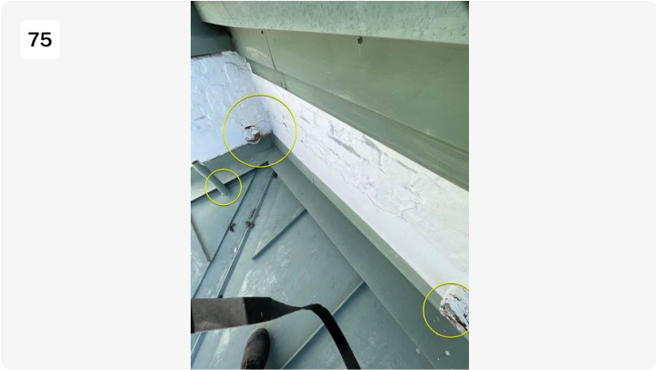
Clogged outlets, and no pipe flashing installed is observed on SS metal roof
