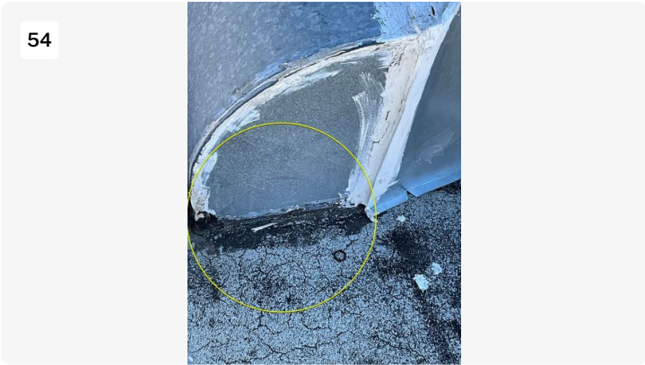
BUR membrane is cracking & tearing
