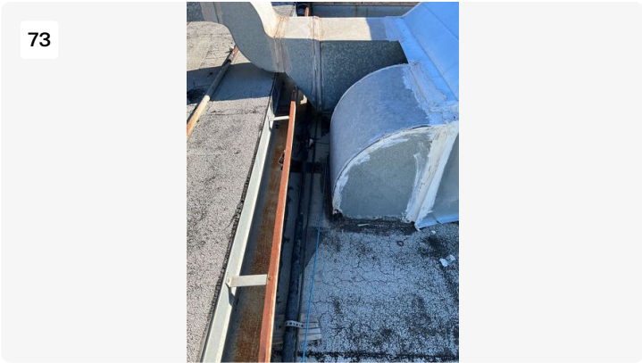
AC ducts with repair material observed
