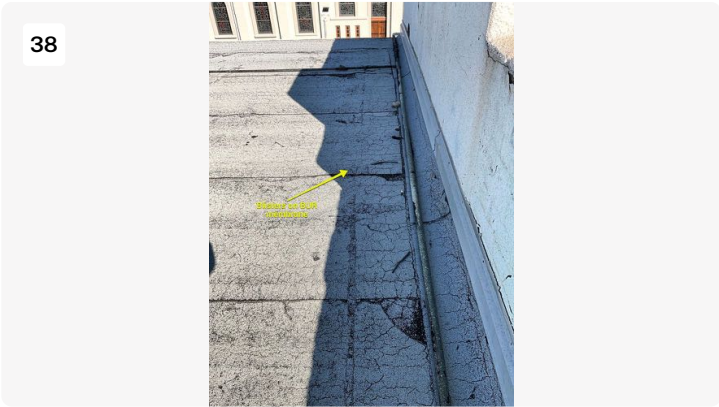
Roof blisters on BUR membrane
