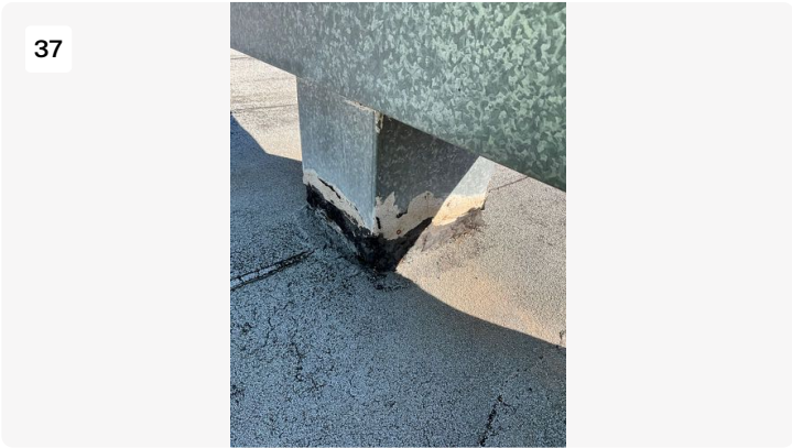
BUR membrane coming apart at roof penetration
