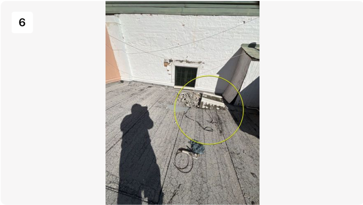
Debris on roof
