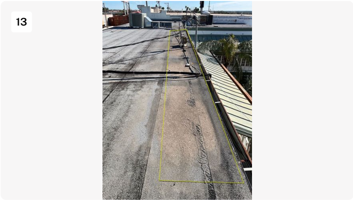
Ponding water stains observed
