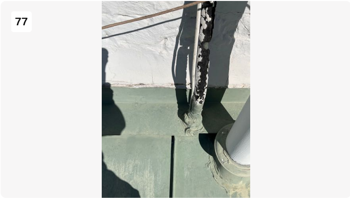
Previous repair material is observed
