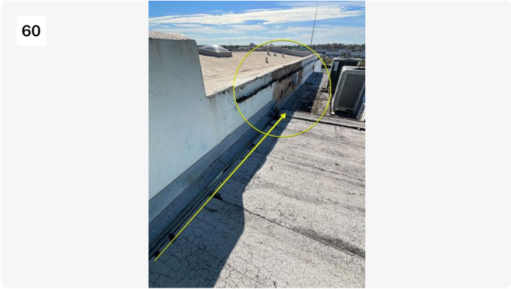
BUR membrane is detaching at the base, in addition the parapet wall is severely peeling & cracking
