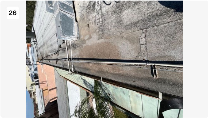
Discoloration, water ponding stains, and severely worn BUR membrane observed
