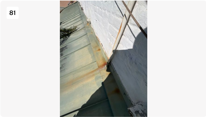
Voids on counter flashing sealant
