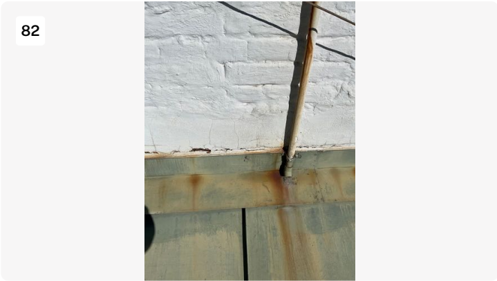
Voids on counter flashing sealant
