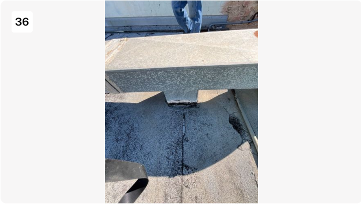
BUR membrane coming apart at roof penetration
