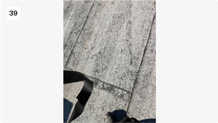
Voids at seams/joints of BUR membrane
