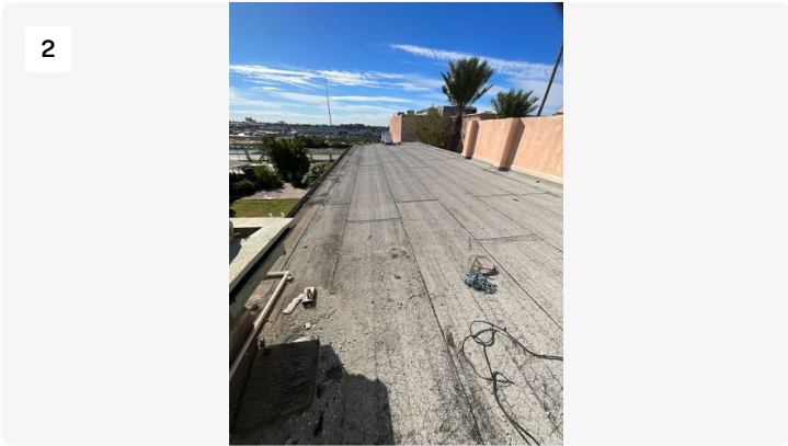
Debris on roof
