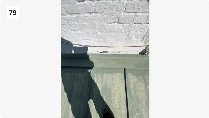
Voids on counter flashing sealant
