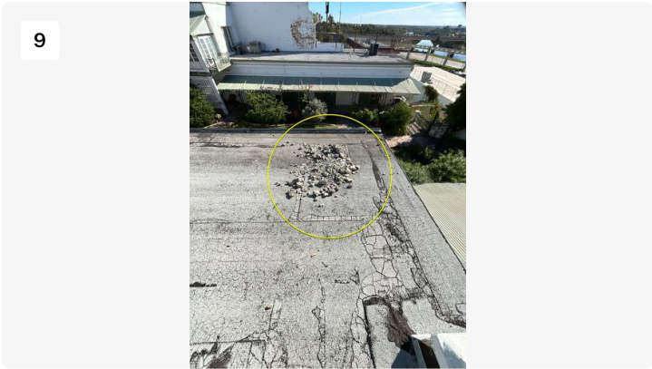
Debris on roof
