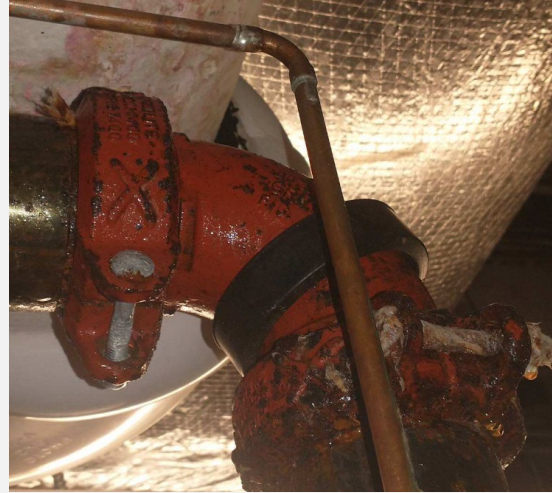
Failing CHW fitting at Admin
