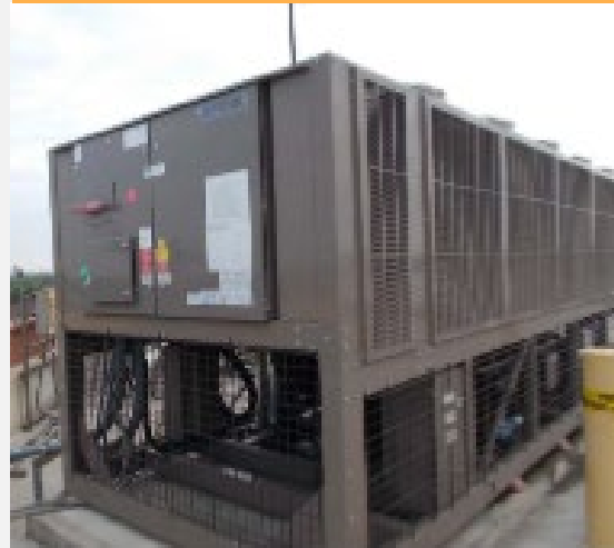
AC Chiller at the Admin
