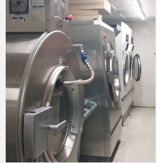
Laundry Equipment in the Jail
