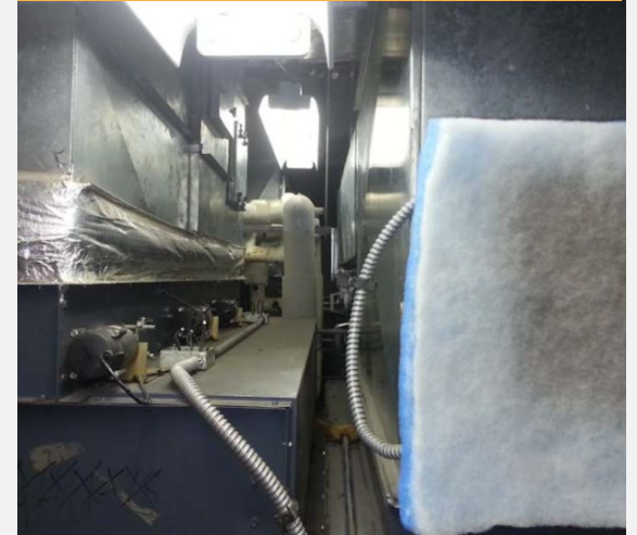
MZ AHU at the Justice Center
