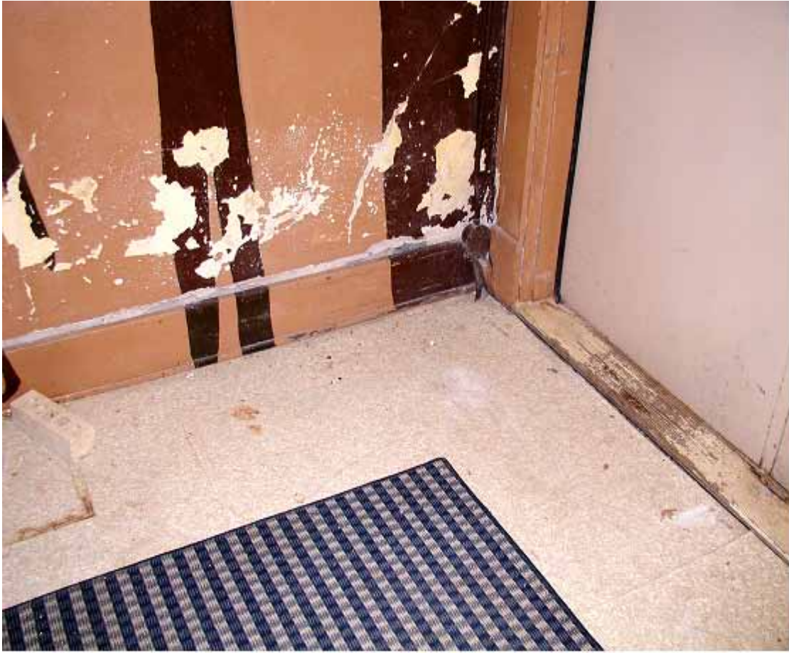
AREA OF WEAK FOUNDATION
