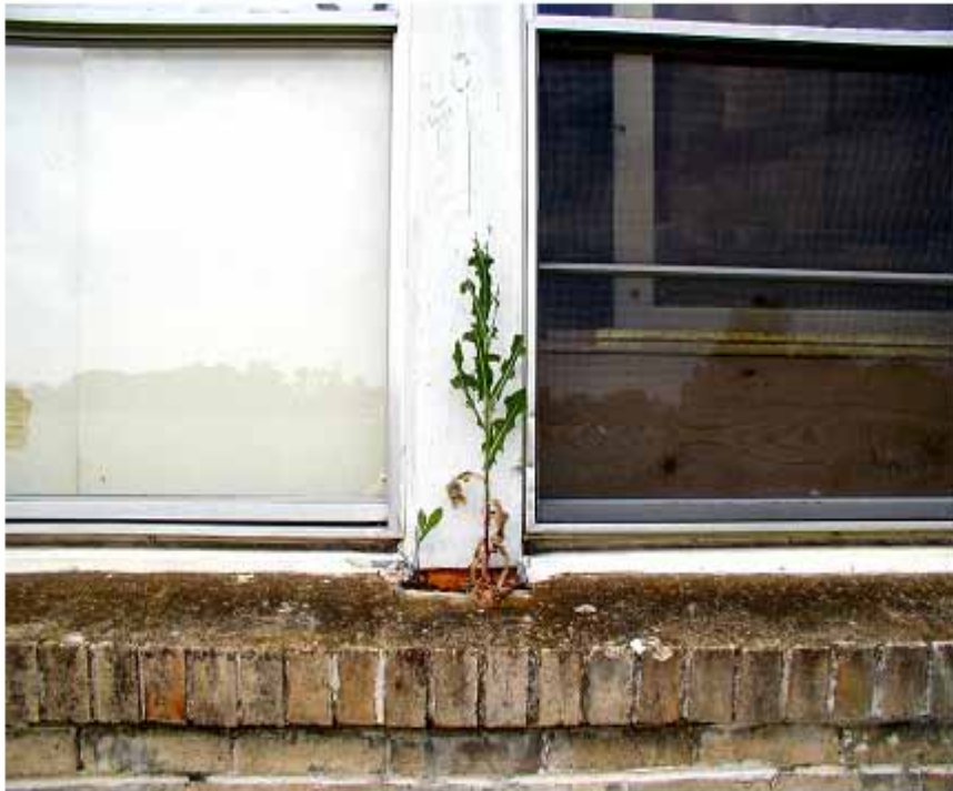
VIEW OF EXTERIOR REPAIRS NEEDED
