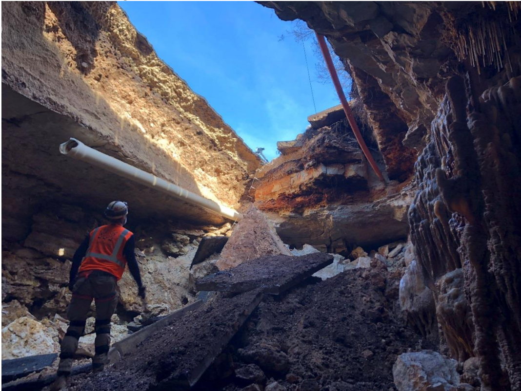
Photo 1. View of collapse area facing north.
