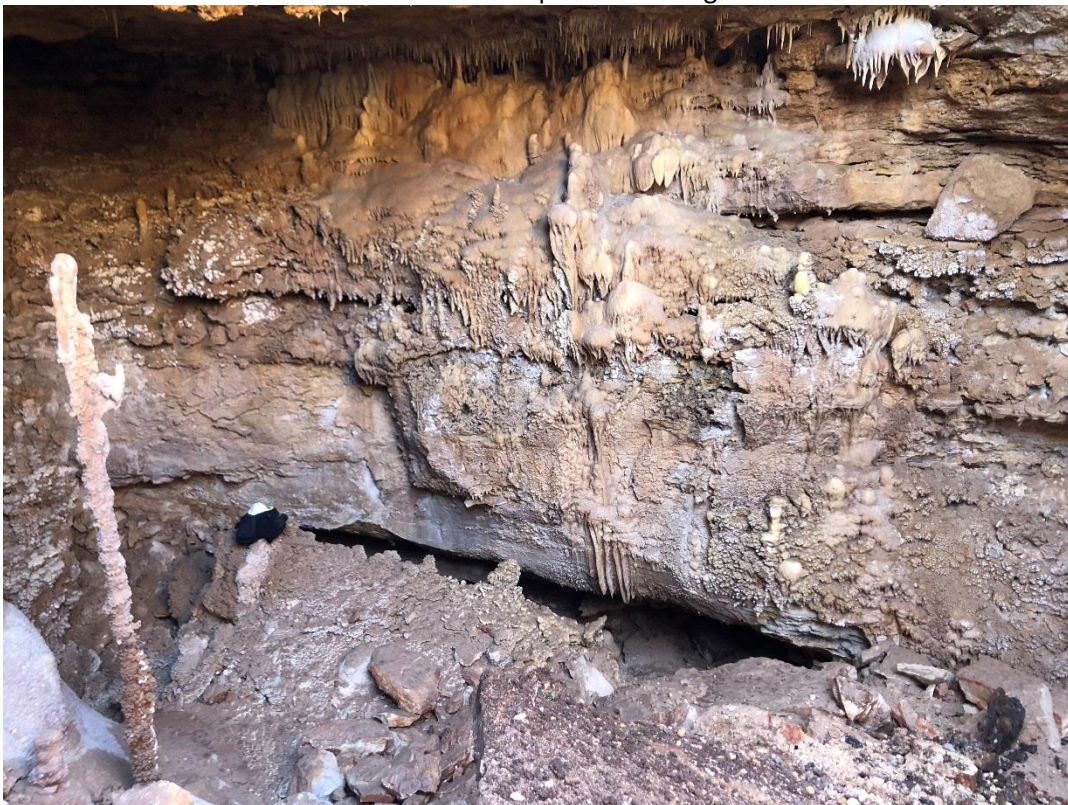
Photo 2. South wall of collapse area with drain.
