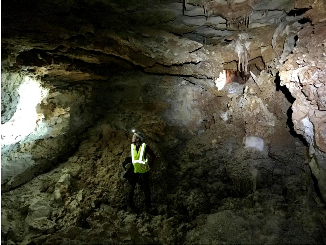
Photo 7. View of second chamber facing west. Light from the collapse area can be seen at upper right.
