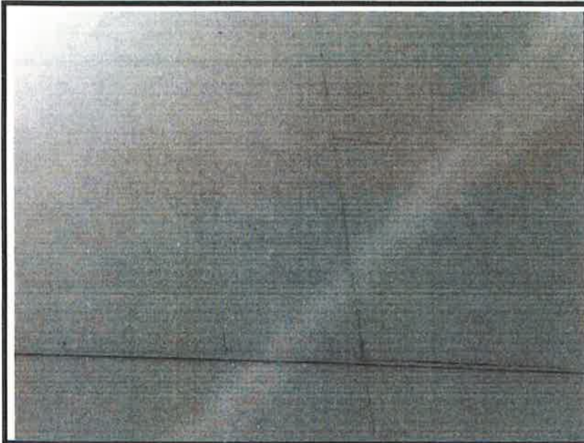
Photo No. 3 Example of open siding joint between panels Example of cracked panels
