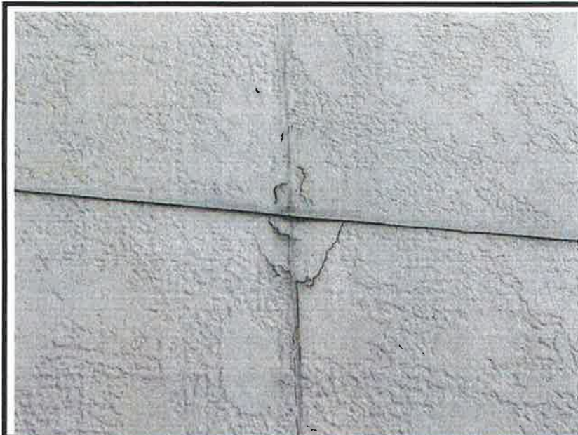
Photo No. 1 Example of damaged siding.
