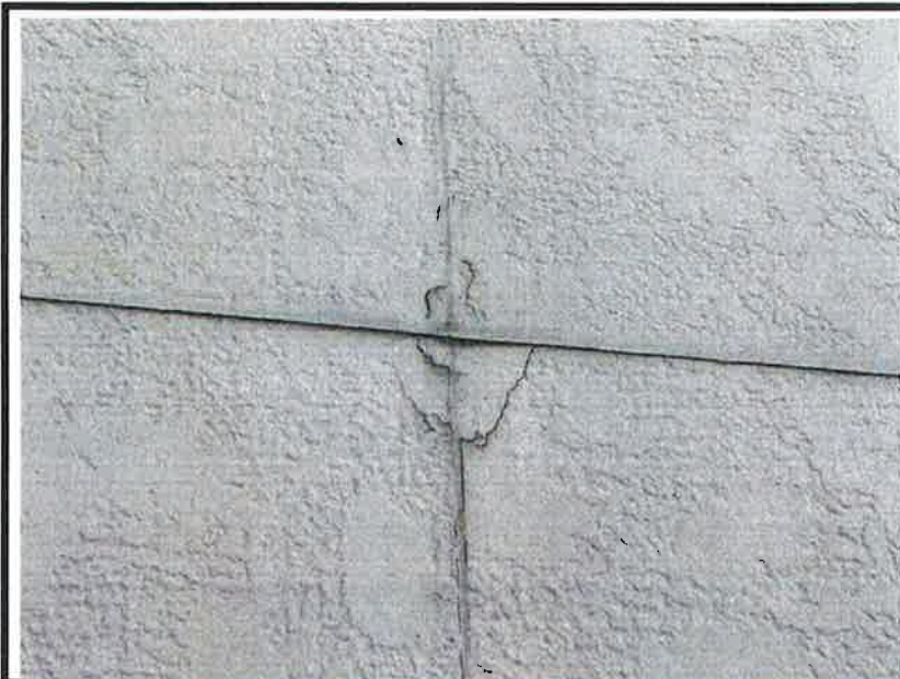
Photo No. 1 Example of damaged siding.
