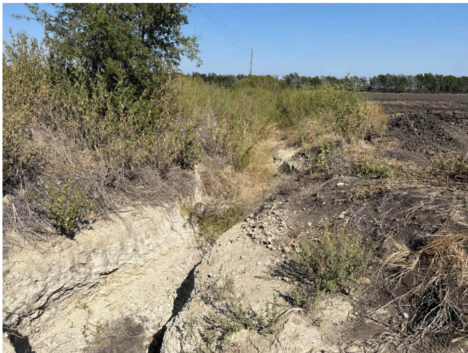
Photograph 8 (PP08): View of erosional wash between agricultural fields, facing upstream and west.
