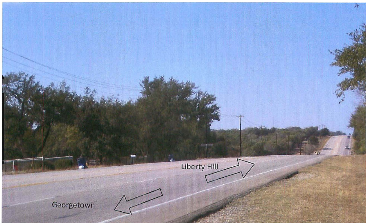
Figure 24. Existing Condition: Cedar Hollow Sight Distance
