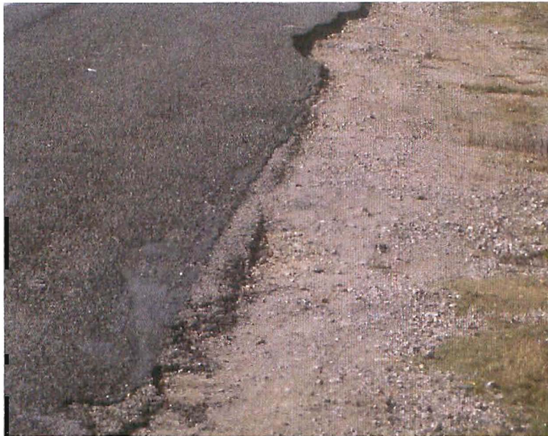
Figure 32. Existing Condition: Typical Shoulder Edge, Burnet Co. Line to Liberty Hill High School Driveway
