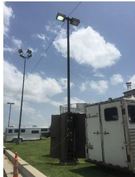
LIGHT POLE W/ UTILITIES
