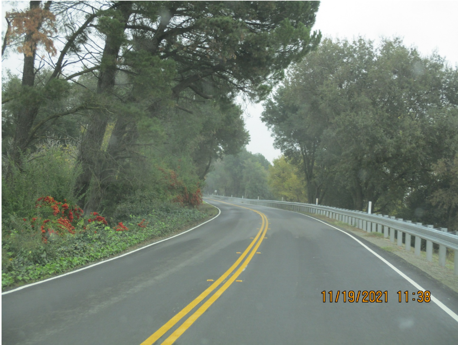
South of Freeport Bridge South River Road, Guardrail and Cape Seal – Photo 1
