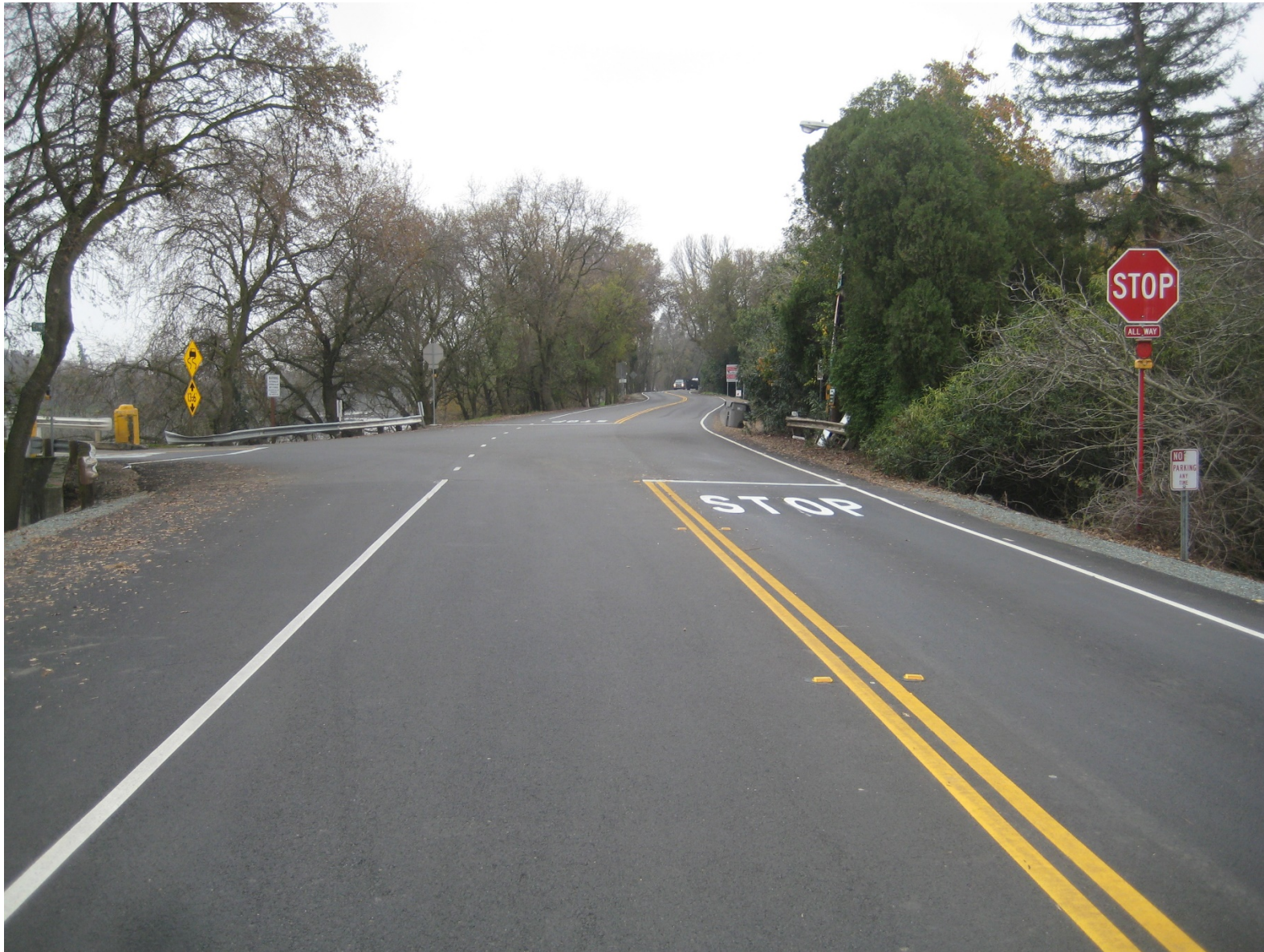
At Freeport Bridge, South River Road, Cape Seal to the South, Cold in Place Recycling and new Asphalt to the North – Photo 4
