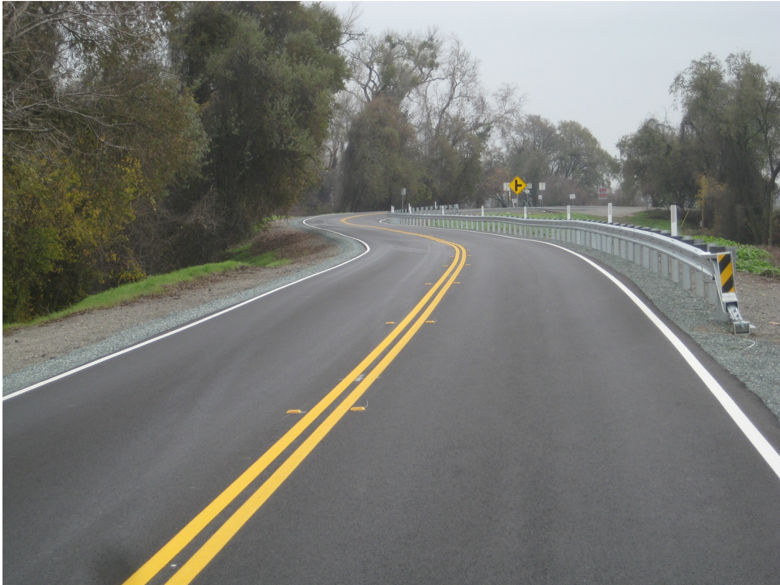
Babel Slough Intersection South River Road, Guardrail and Cold in Place Recycle with new Asphalt – Photo 5
