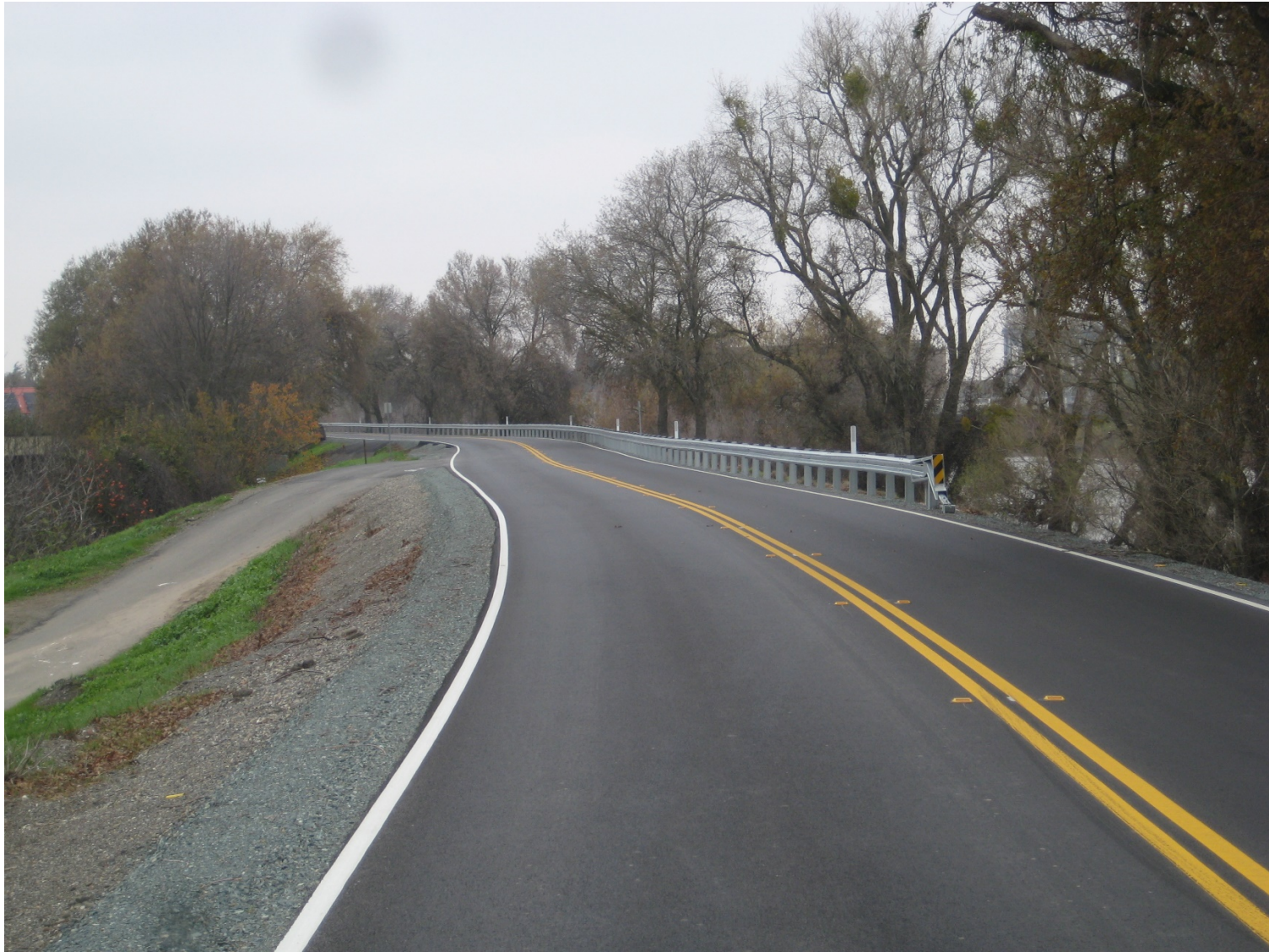
North of Freeport Bridge South River Road, Guardrail and Cold in Place Recycle with new Asphalt – Photo 6
