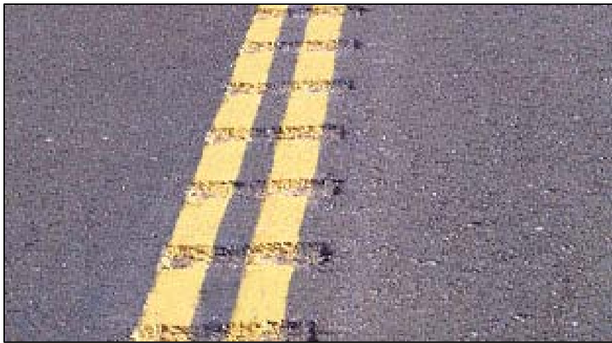
Figure 2 - Centerline rumble stripes on levee roads (Old River Rd & South River Rd)
