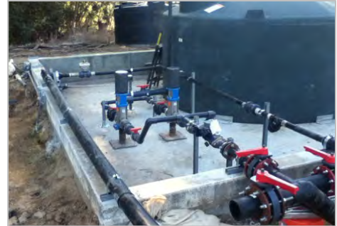
SCS constructed, operated, monitored, and maintained this Leachate Control System at the Crazy Horse Canyon Landfill.
