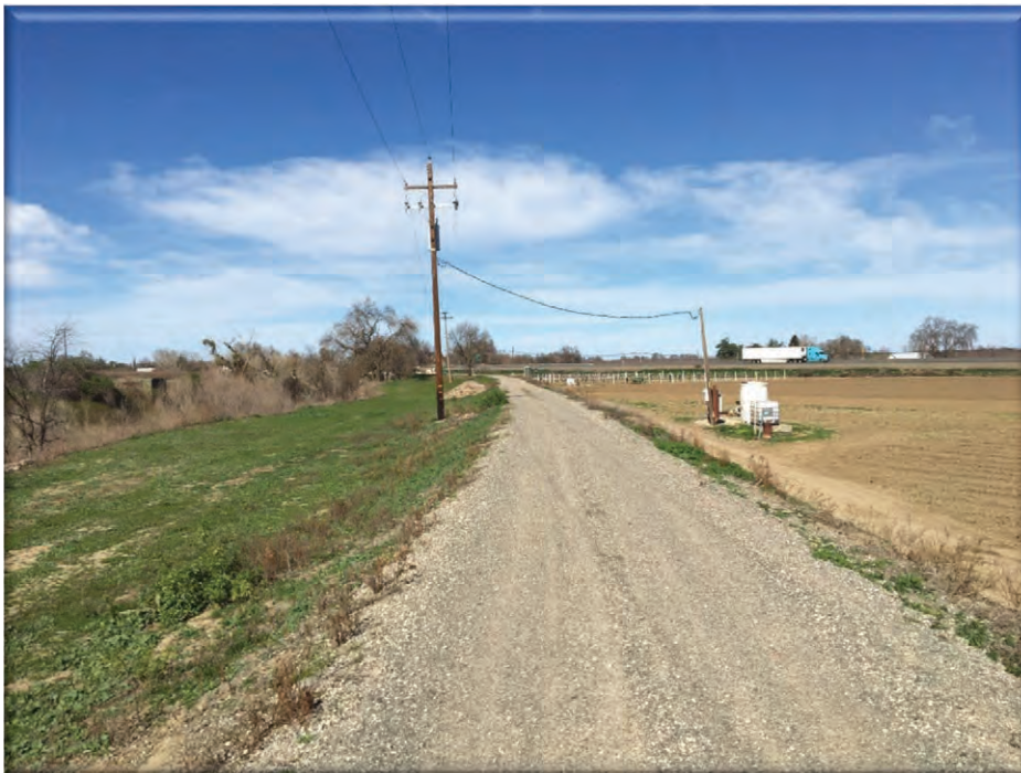
Plate 2. Looking east along the levee road east of County Road 18 toward Interstate 5. The levee rehabilitation project includes the graveled levee road and approximately 20 feet on both sides of the levee road.
