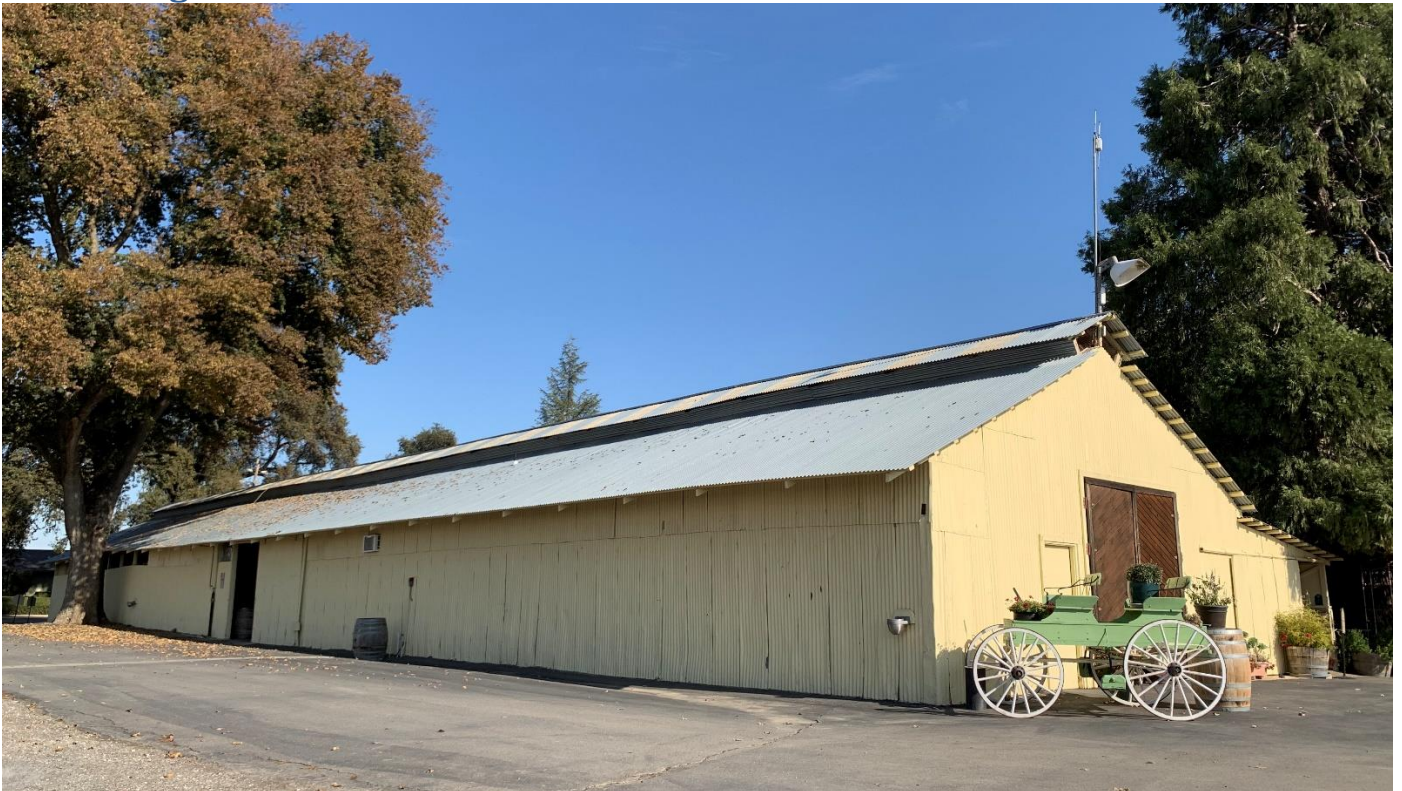
Figure 26: West and South façades of the Barn at Utter Ranch, looking northeast. Photo by Lyn Hooper, 2020.
