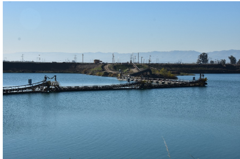
Working Conveyor – from dredge on left to south side of pit and on to plant site
