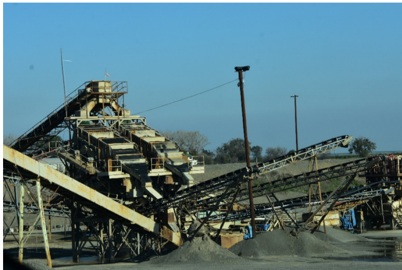
Teichert-Esparto – Plant equipment. Began processing material in
