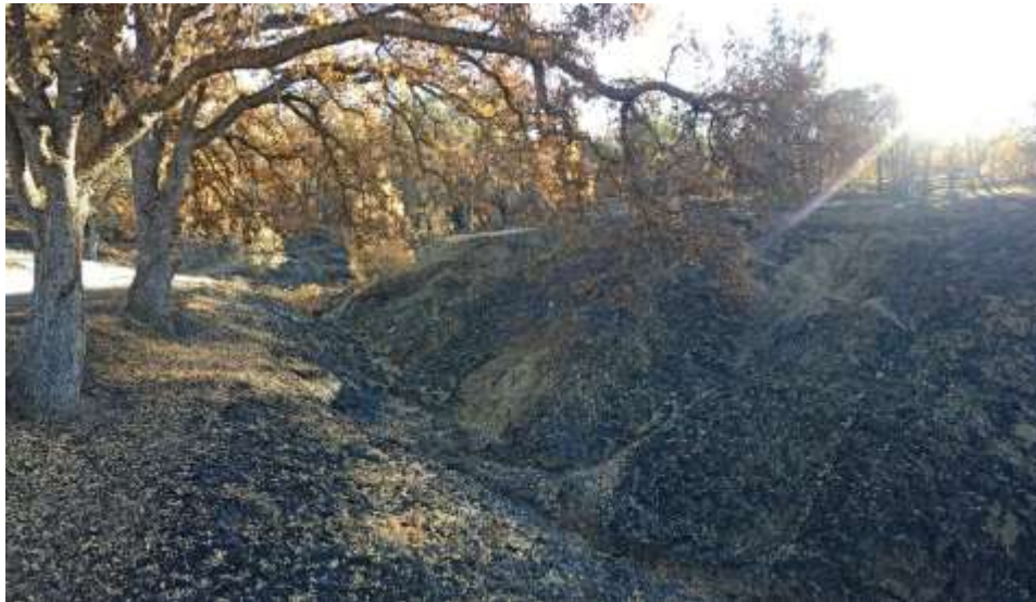
Photo 6: A drainage that was burned in the LNU Lightning Complex Fire, 2020.
