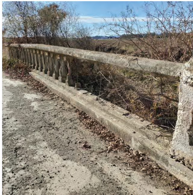
Figure 6. Bridge damage, viewing southwest
