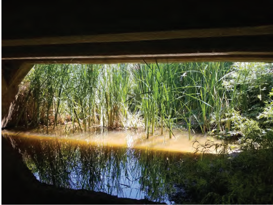
Overview of the underside of the Union School Slough Bridge. Taken facing east.
