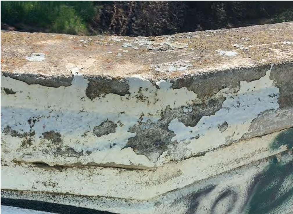
Photo 3. Flaking and peeling paint at northeast corner.
