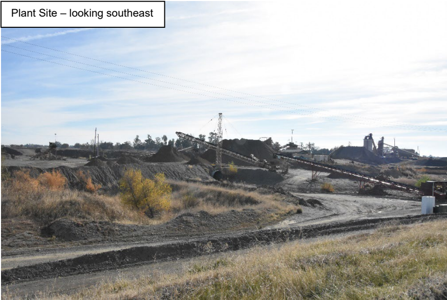
Conveyor from Shifler mine excavation – western side of plant site – looking south
