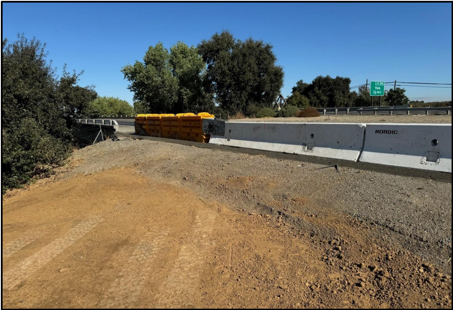
Standing on newly constructed levee prism facing north towards southbound Interstate 5 at the installed shoulder closure objects.
