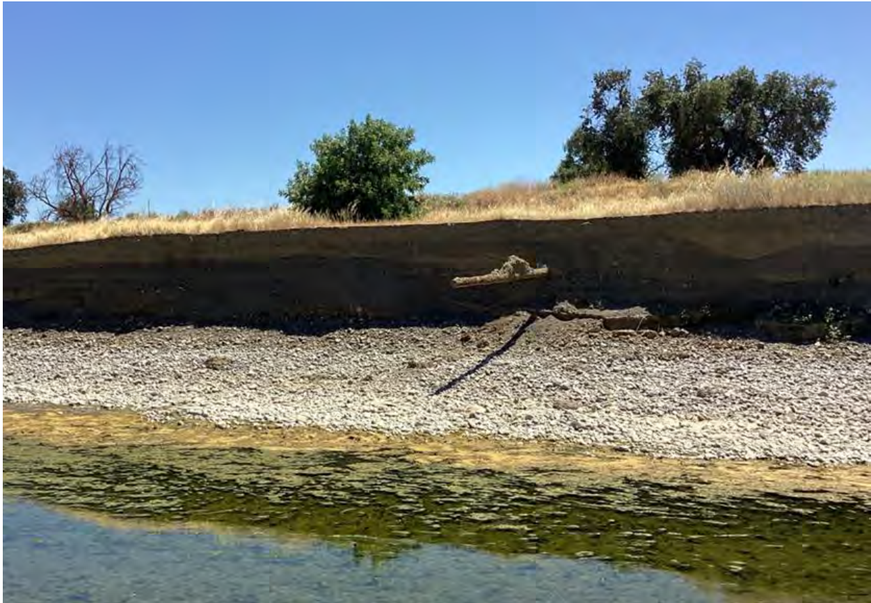
Figure 2-21. Exposed pipe in south (right) bank at River Mile 22.5.
