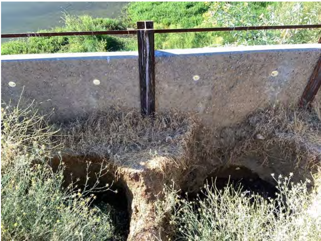
Figure 2-14 View of soil erosion behind Bank Repair Wall at Capay Dam. (2024)
