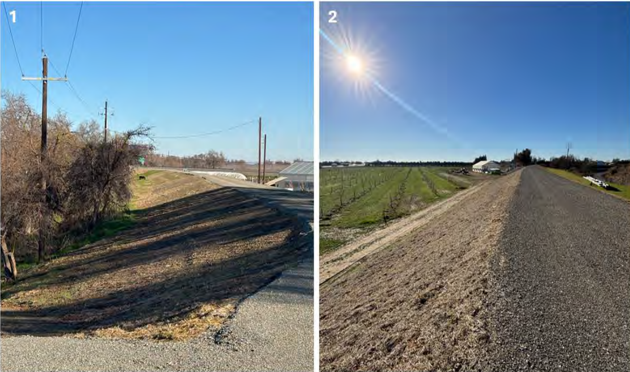
Figure 5. Representative photos showing the completed Huff's Corner Levee Maintenance Project. Photo 1 depicts the waterside slope looking upstream towards I-5. Photo 2 depicts the landslide slope looking downstream. Photos taken January 22, 2025.
