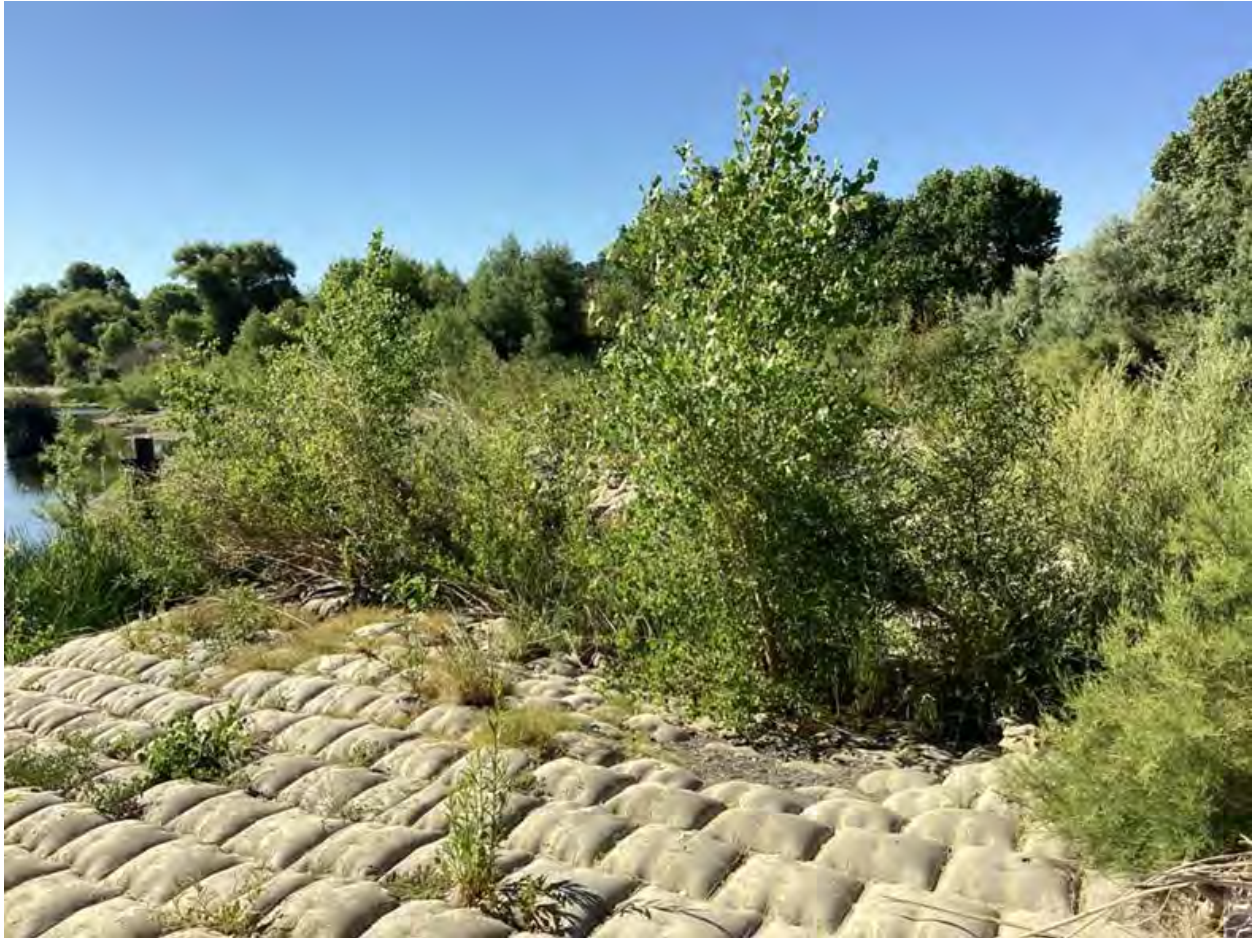
Figure 2-15. Photo showing current state of erosion control blanket at PG&E Palisades site including substantial riparian vegetation growth (2024 Creek Walk).
