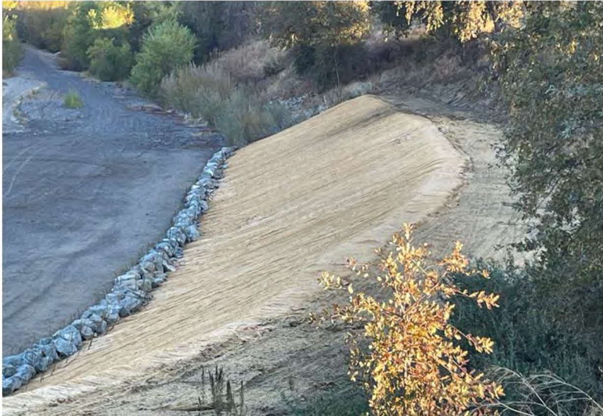
Figure 4. A portion of the completed Huff's Corner In-Channel Repairs Project. Photo taken November 18, 2024.
