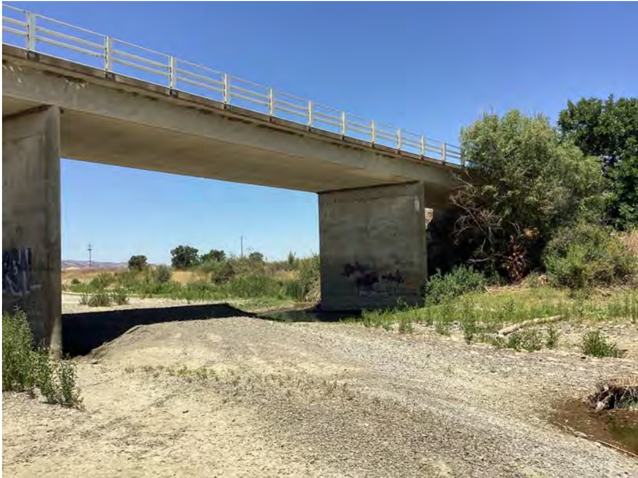
Figure 2-19. Photo from 2024 Creek Walk showing Esparto Bridge piers with no significant change from last year.
