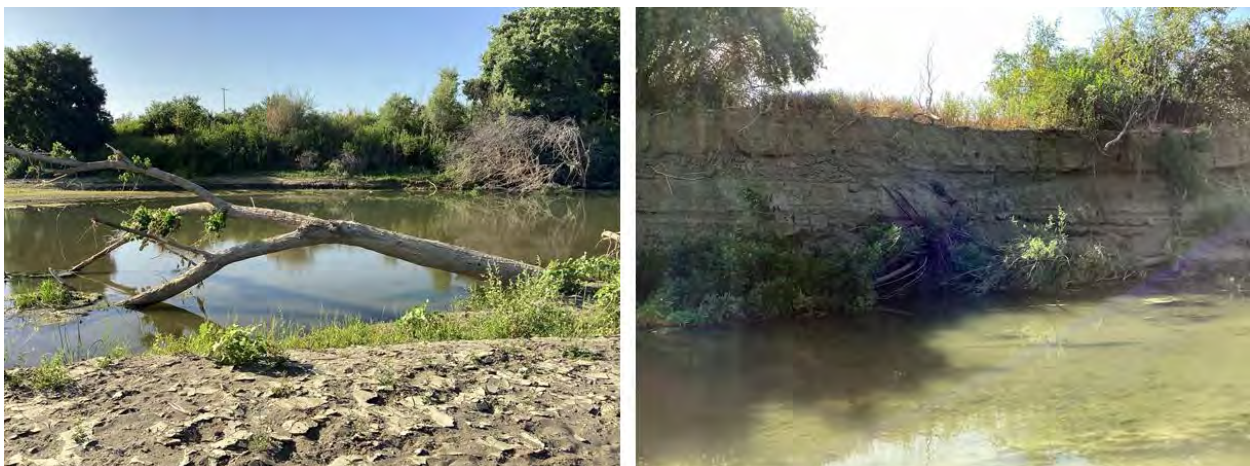
Figure 4-4. Examples of native woody vegetation displaced from banks into the main stream channel by bank erosion resulting from winter 2023-2024 flows in the Hoppin Reach at RM 15.7 (left) and RM 15.0 (right).
