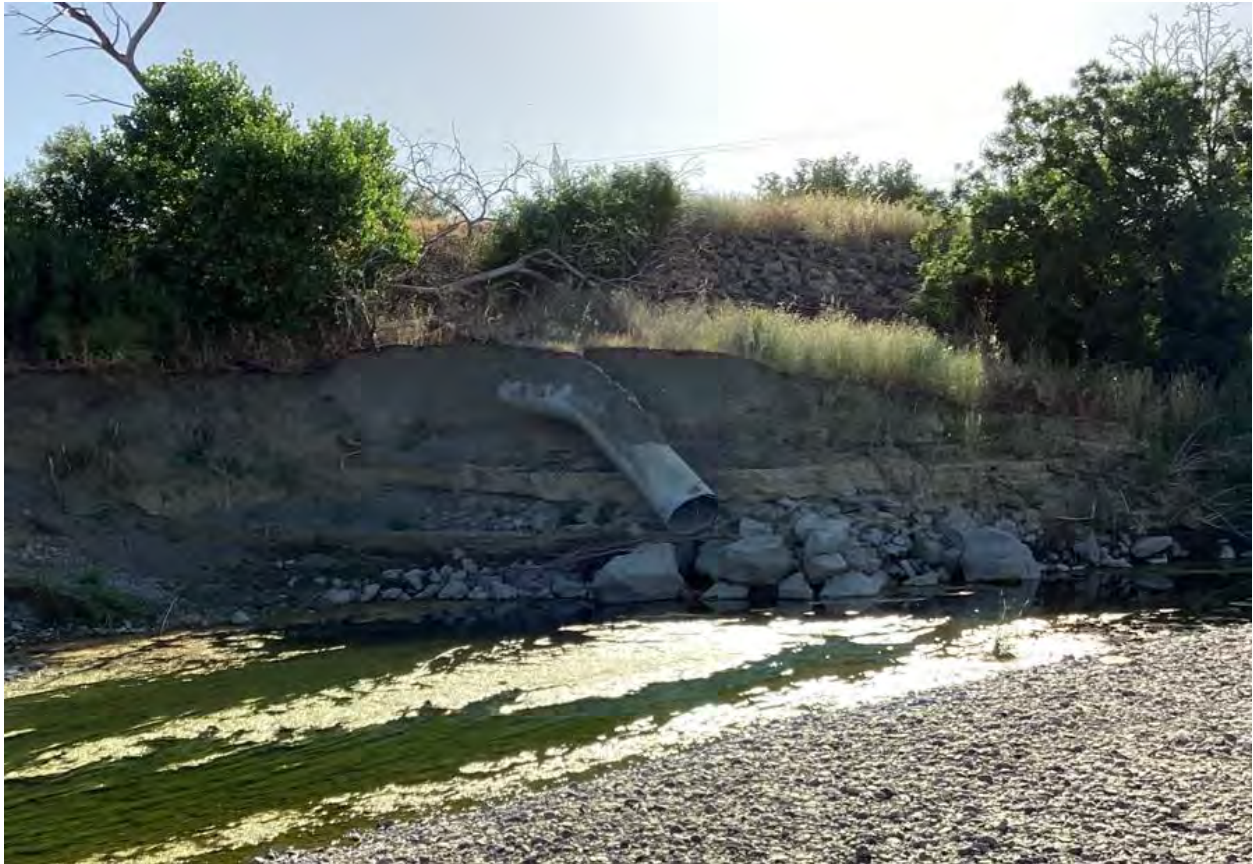
Figure 2-22. Newly eroded bank and exposed pipe at I-505 Bridge.
