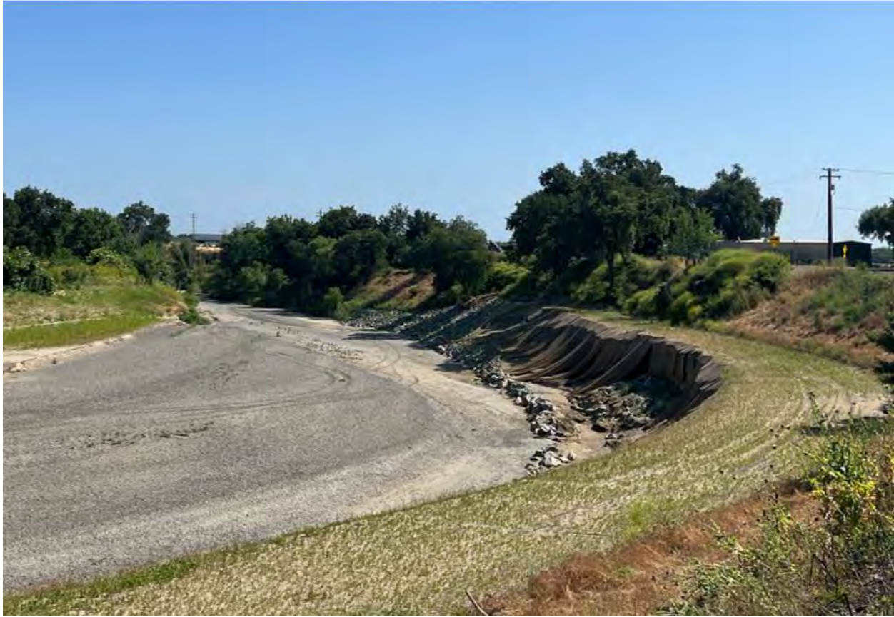
Figure 3. State of the Huff's Corner In-Channel Reconfiguration Project after Winter 22-23 flows damaged the newly constructed right bank terrace. Photo taken June 2, 2023.
