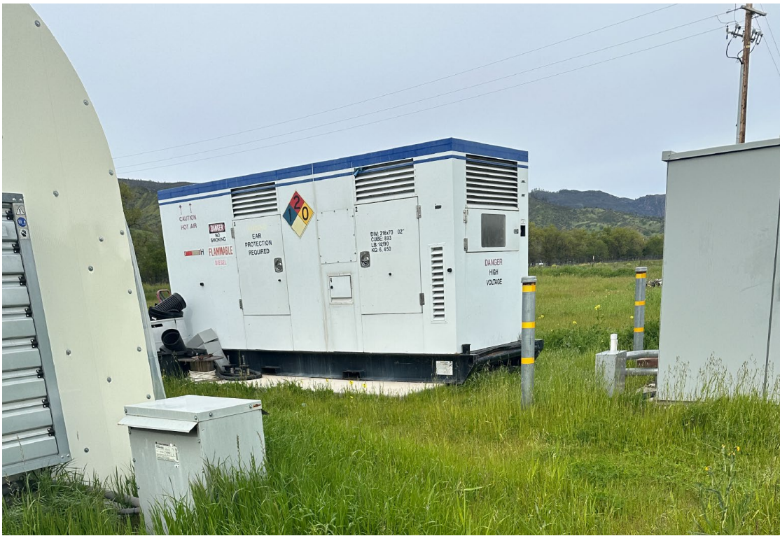
Generator installed without permits (opposite side) (3.20.25)
