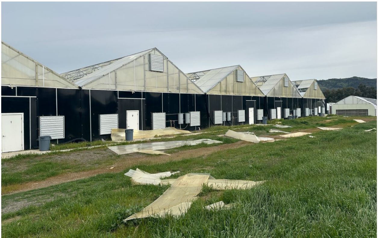
Damaged greenhouses and debris (3.20.25)
