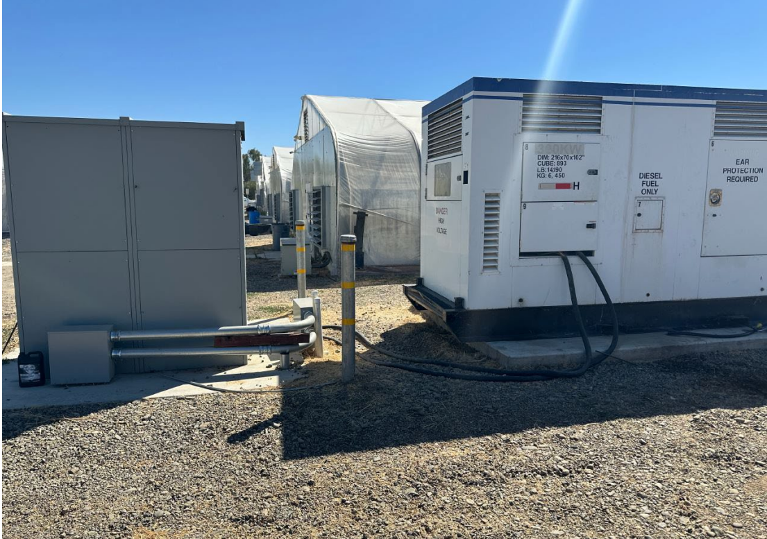
Generator installed without permits (3.20.25)
