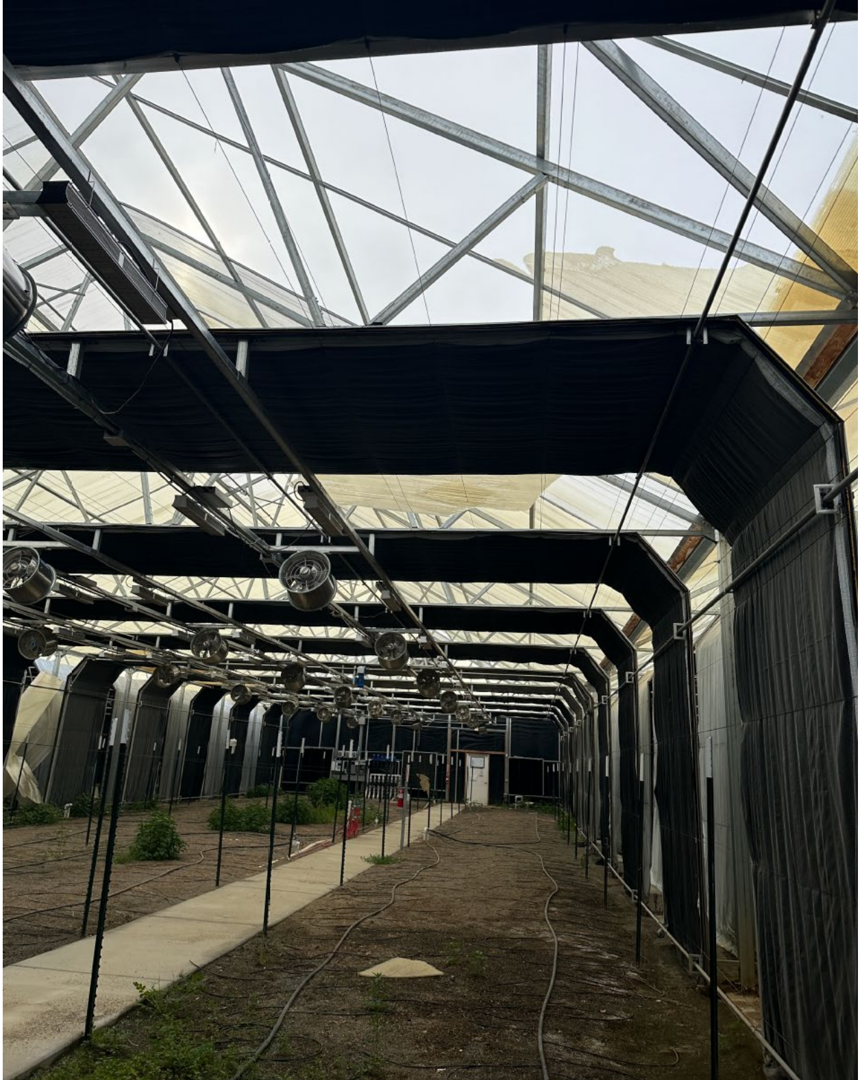
Inside damaged greenhouse (3.20.25)
