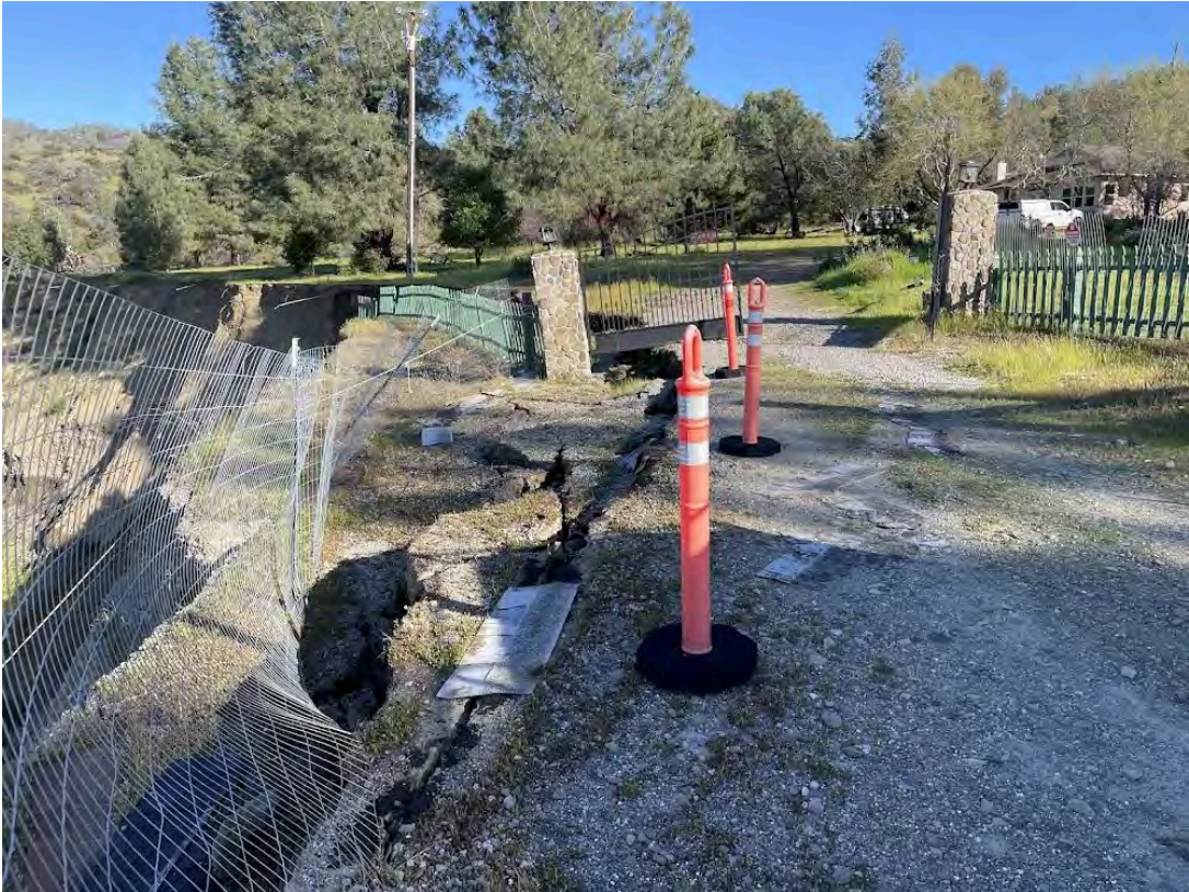
Landslide- March 2024 - Loss of fence, driveway, at least a 15 foot wide shelf along the length of the property
