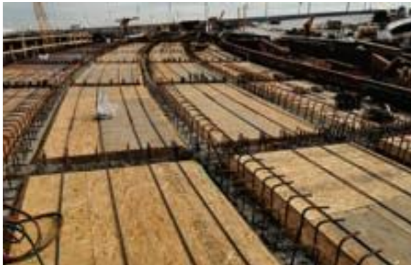
Rob and Ryan will verify deck thickness and grades prior to placement of reinforcing steel
