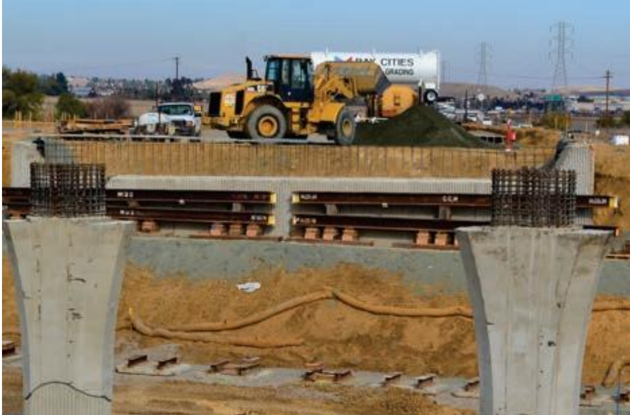
The Mark Thomas Team are experts in cast in place concrete box girder bridges
