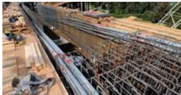
Careful attention must be paid to the concrete consolidation around prestress ducts and anchorages
