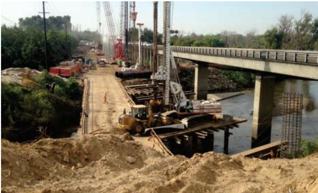
Michael, Indy, Rob, and Ben have over 100 years of combined experience with CIDH piling installation.
