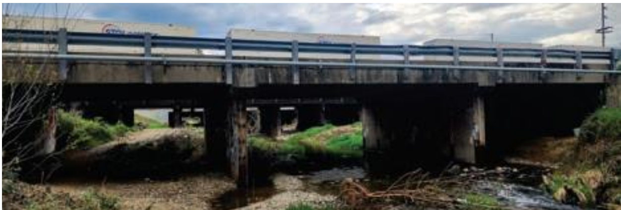
Ryan performed construction inspection services on the Eastside Road Bridge over Olney Creek in Redding
